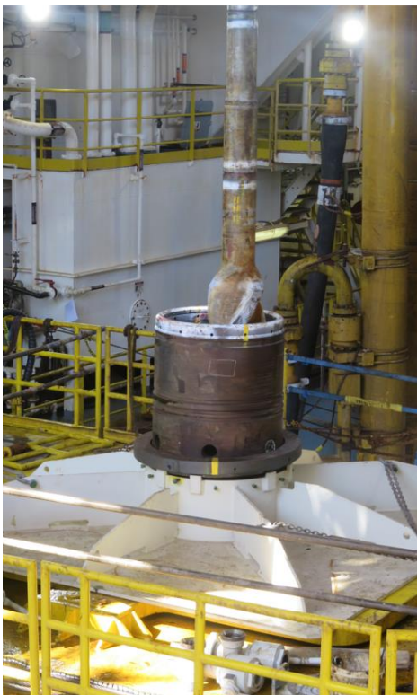
Installation of the bottom hole drilling assembly within the well head housing on the mudmat.
